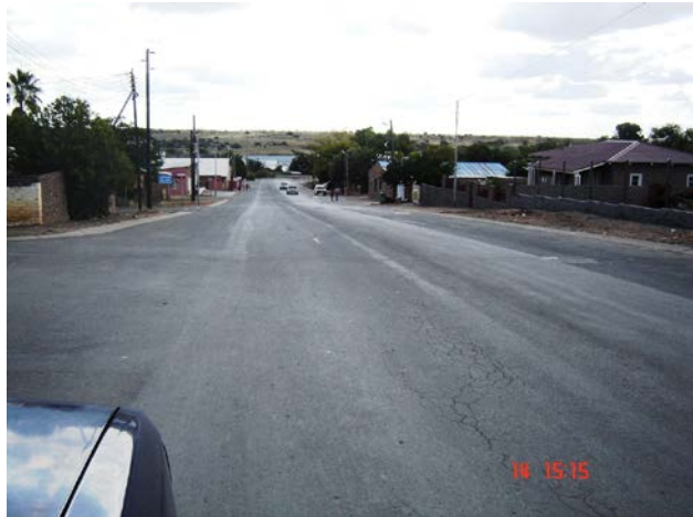
General Cracking of street surface
