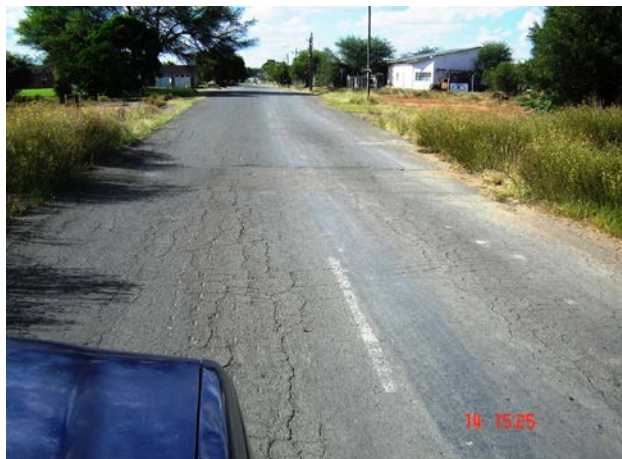
Failure on road where ponding occurs
