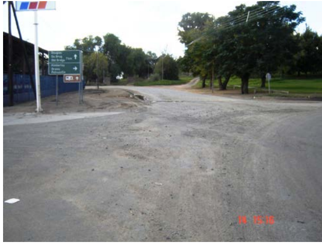
Storm water drainage problem
