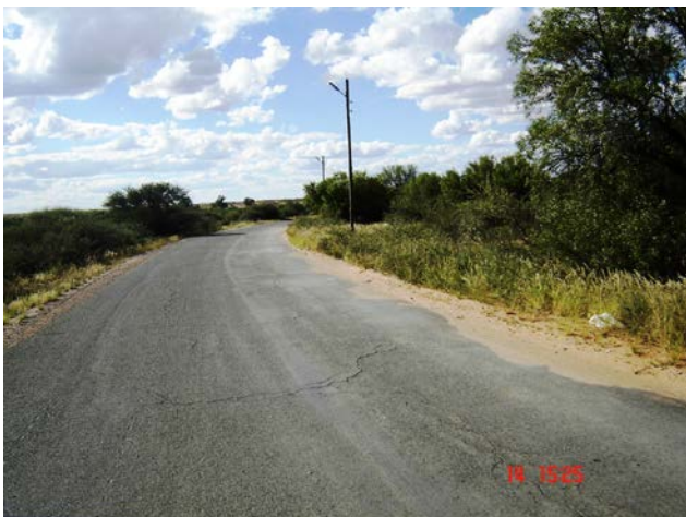
Cracks and drainage problems
