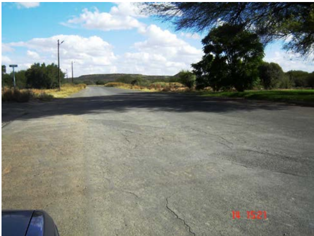
Cracking of surface
