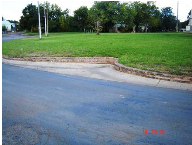
Surface failure and storm water drainage
