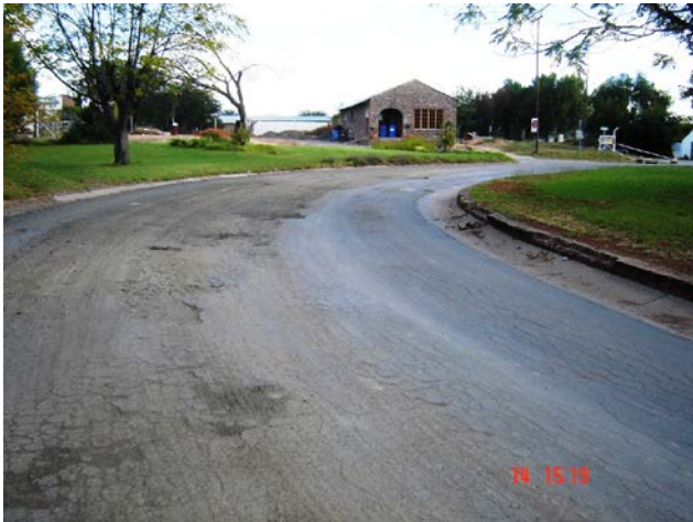
Surface failure around traffic circle
