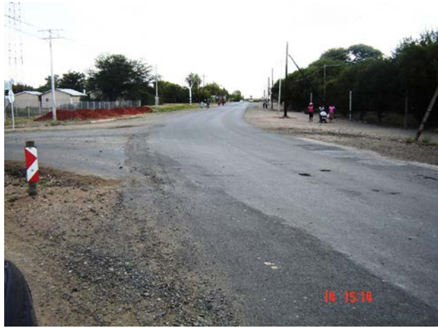
Potholes and general condition
