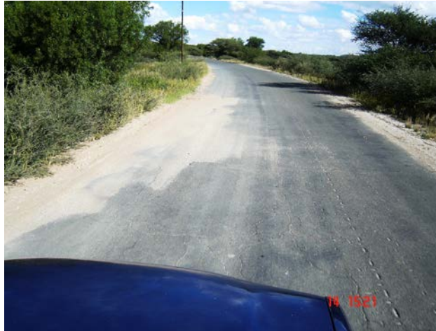
Poor drainage results in ponding of water
