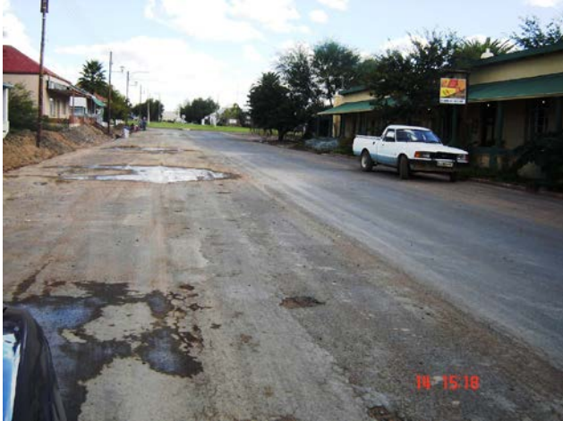
Poor condition of Main street
