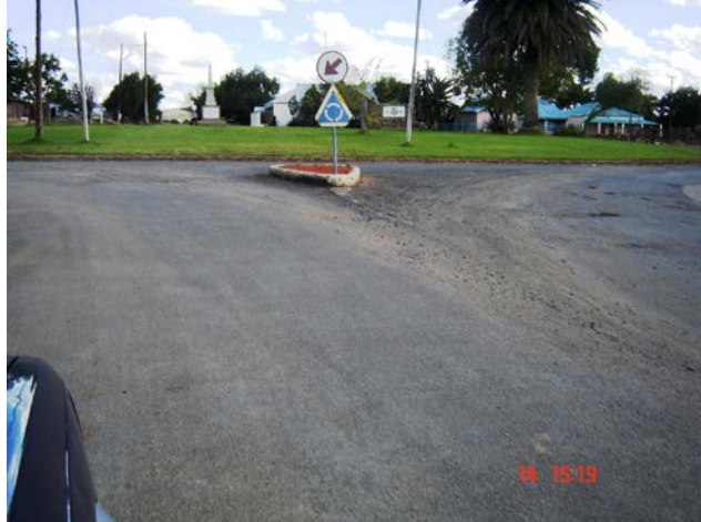
Surface failures at traffic circle exit
