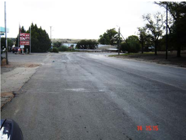
Surface failure / rotten concrete canals
