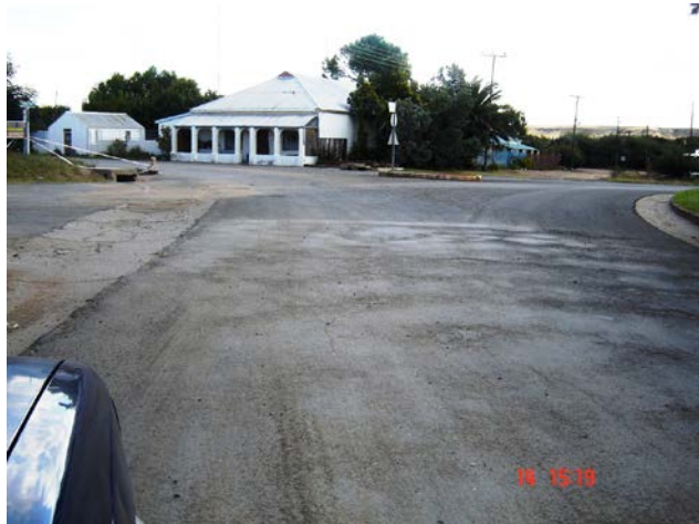
Poor condition of surface around circle
