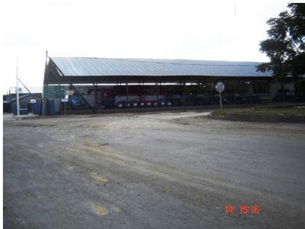
Storm water problems
