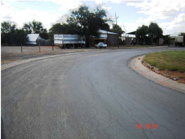
Seal cracks around circle
